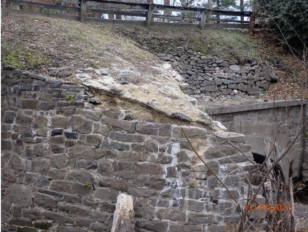
Inlet Side View of Missing Stone on Buttress between the Culvert and Aqueduct – 2021
