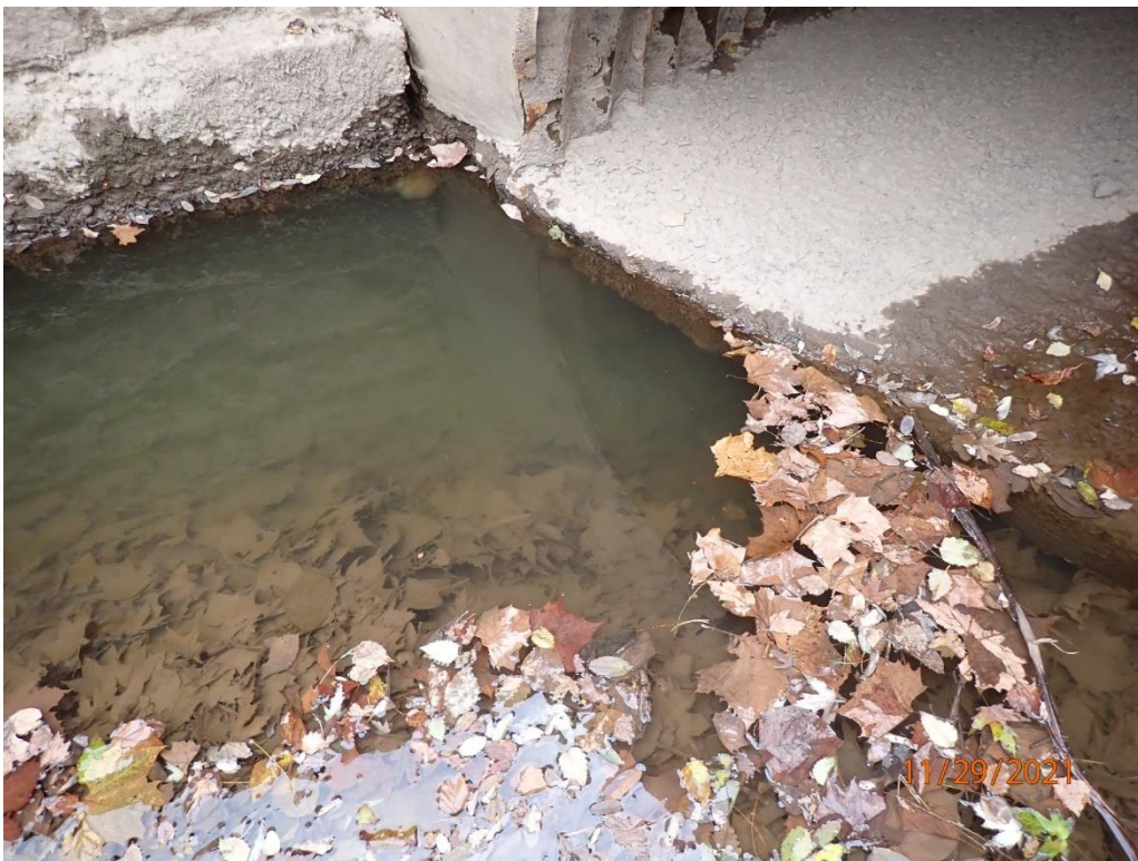
Undermining Beneath the Concrete Floor Slab at the Inlet of Culvert – 2021
