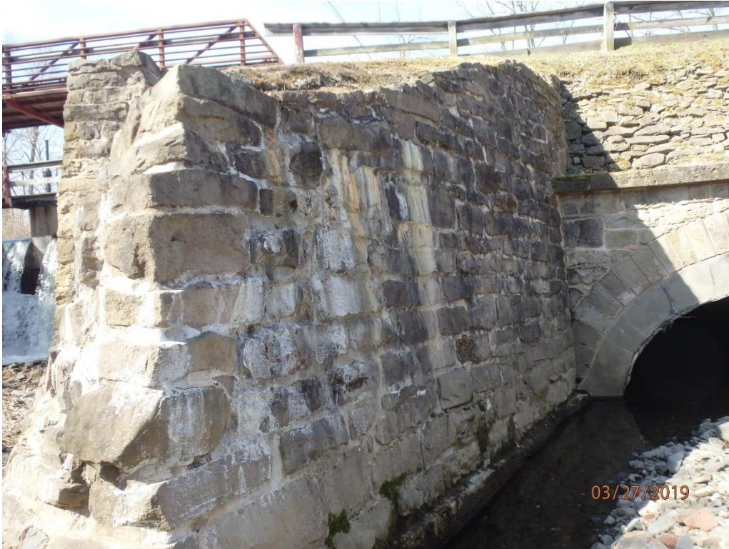
Culvert Inlet Stone Buttress Efflorescence – 2019
