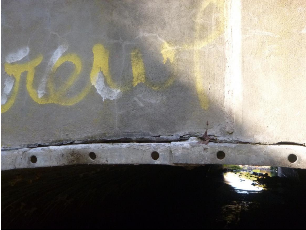
Corroded Corrugated Steel Pipe Liner (Culvert) – November 5, 2025
