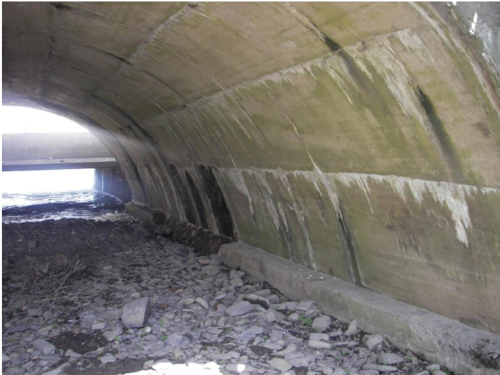
Efflorescence and Wet Spot Inside the Aqueduct – 2006
