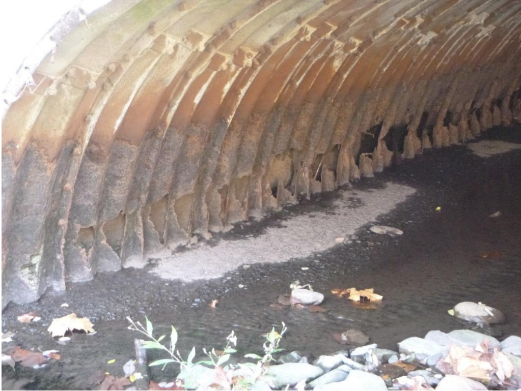
Corroded Corrugated Steel Pipe Liner (Culvert) – November 5, 2025
