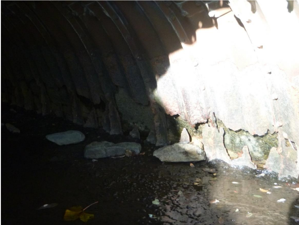
Corroded Corrugated Steel Pipe Liner (Culvert) – November 5, 2025
