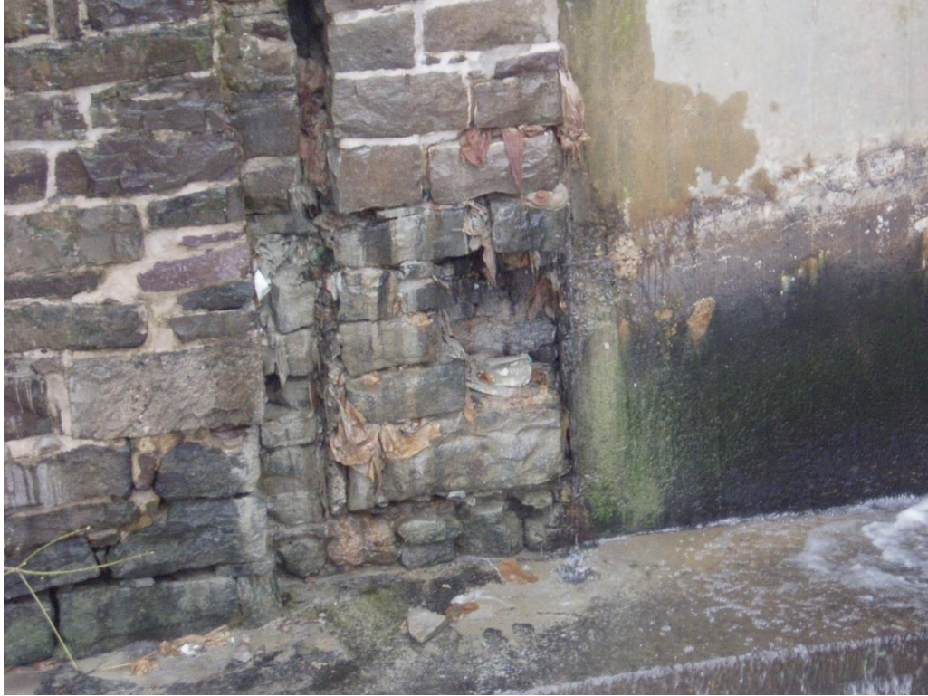
Missing Stone / Deterioration on the Aqueduct (Upstream) – 2005
