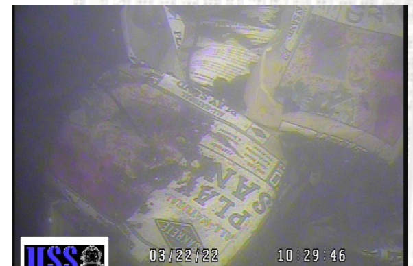
Sand bags under gate
