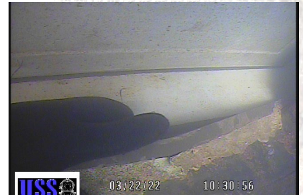
Seal broke free in the right corner
