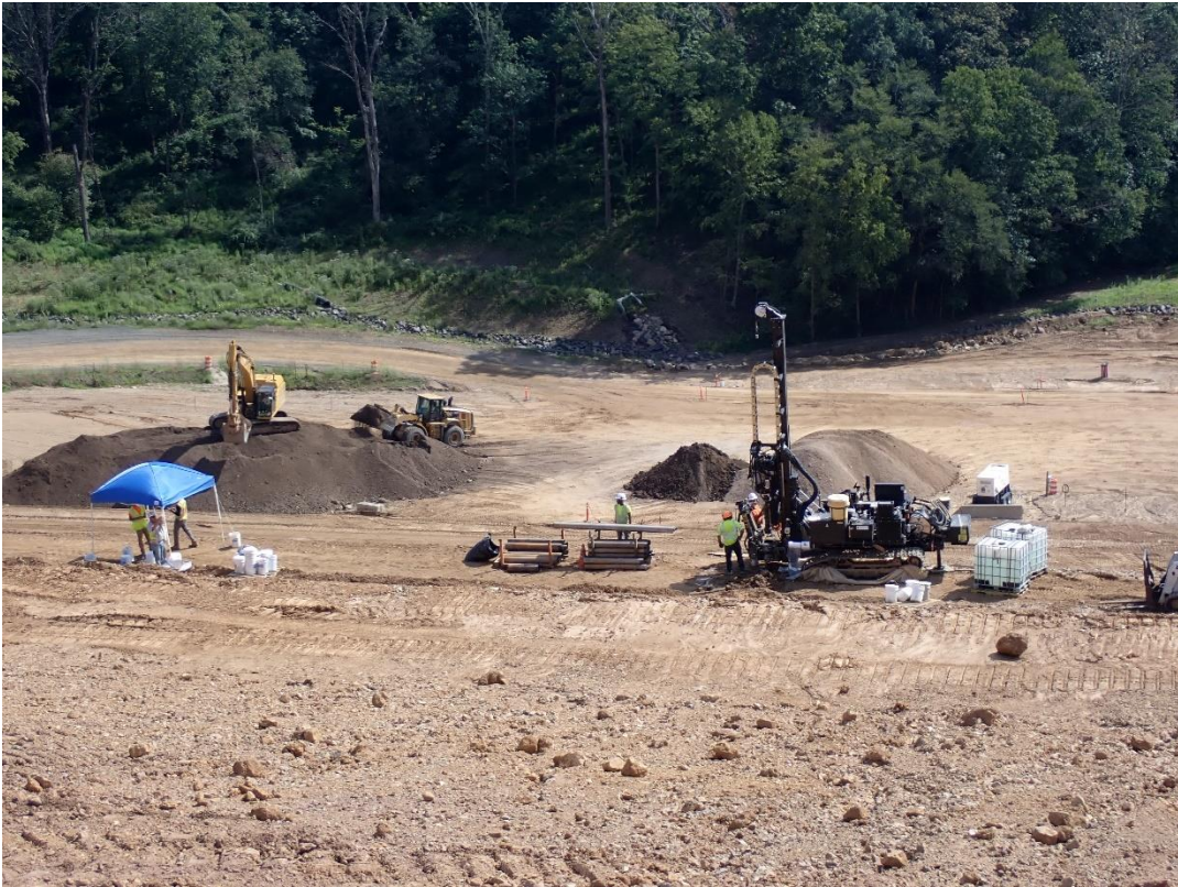
Restoration work progresses at the South Dam - spreading topsoil (L) and installing dam instrumentation (piezometer) (R)
