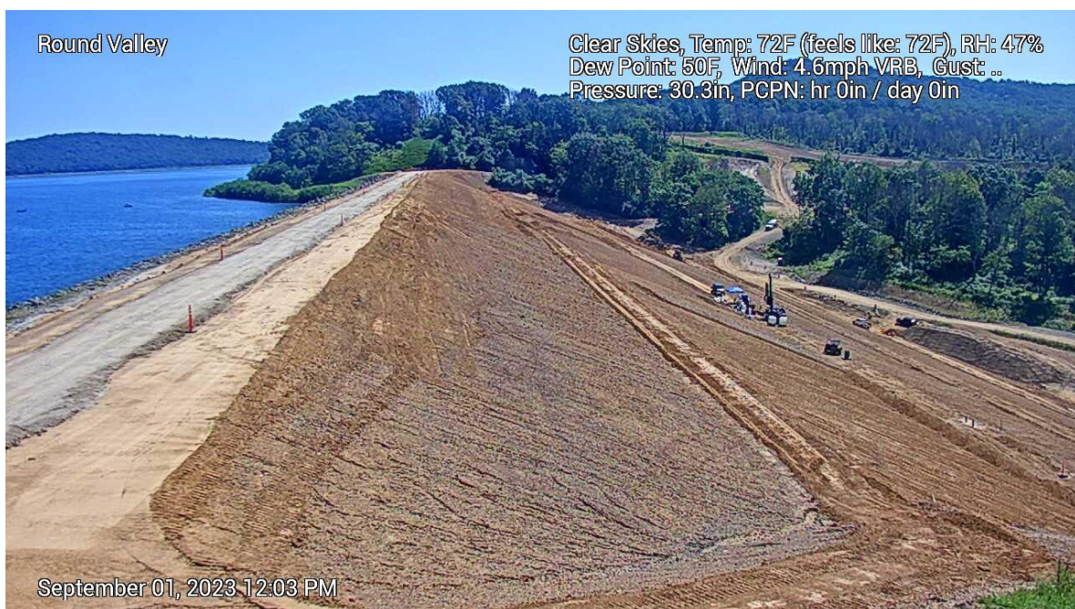
Major earthwork completed to crest elevation at the South Dam – topsoil, seeding, and paving to follow
