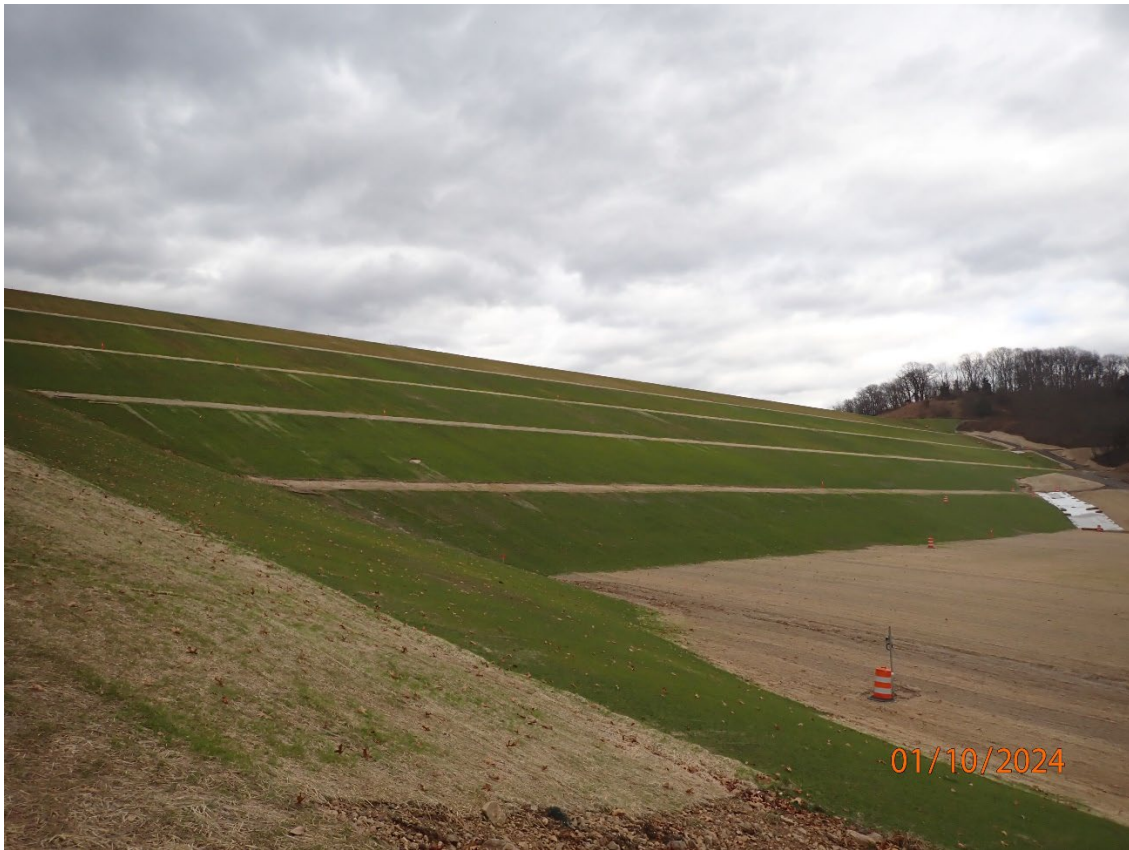
Vegetation has been reestablished on the slope of the South Dam. Minor restoration work continues.
