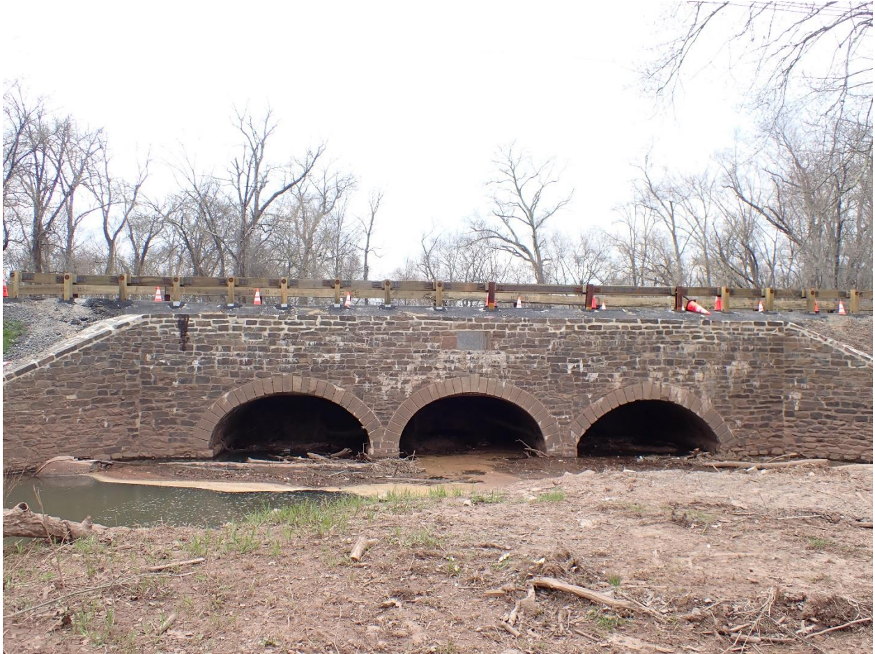
View of Culvert Inlet. Repointed stonework on headwall and within culvert. Repaved, restriped, and new guiderail installed on Canal Road (above)
