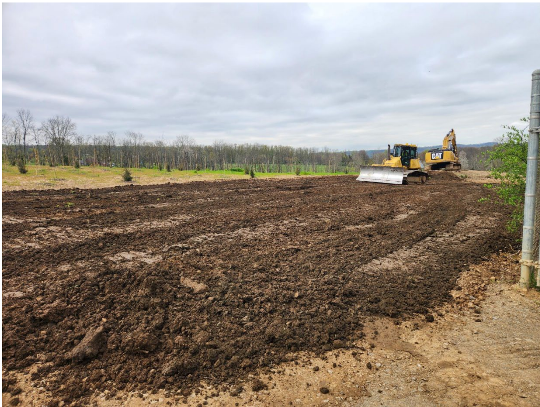
Contractor restoring areas that were used for staging and stockpiling during construction. New tree plantings in reforestation areas can be seen in background.
