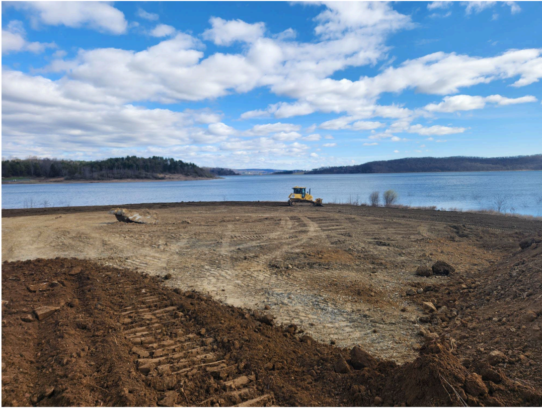
Contractor restoring areas near the South Dam that were used for staging and stockpiling during construction.
