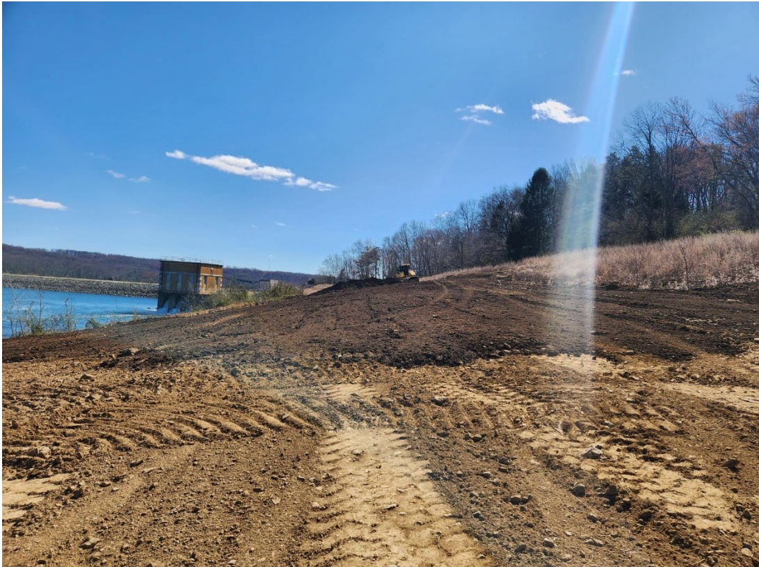
Contractor restoring areas near the South Dam that were used for staging and stockpiling during construction.
