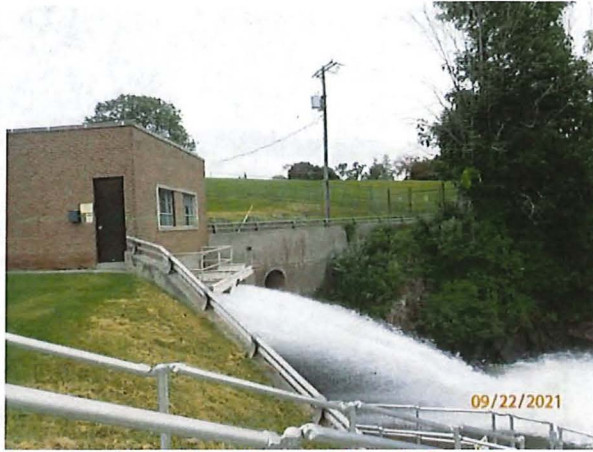
Spruce Run Vault. Howell Bunger Valves in Operation
