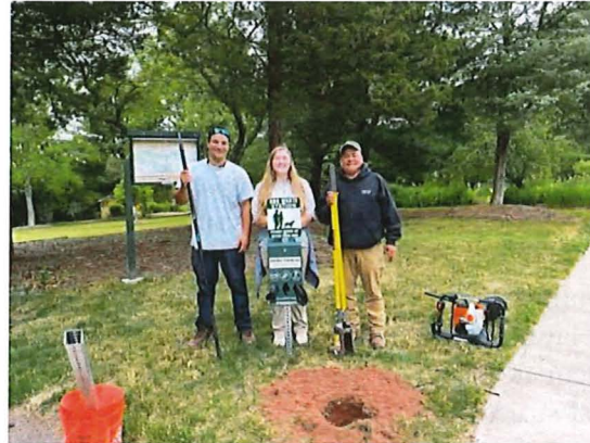
Hillsborough Township Pet Waste Station
