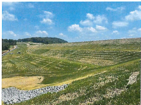
Major earthwork was completed at the North Dam in the summer of 2022. Restoration work, including topsoiling, paving, and installing permanent instrumentation is ongoing.
