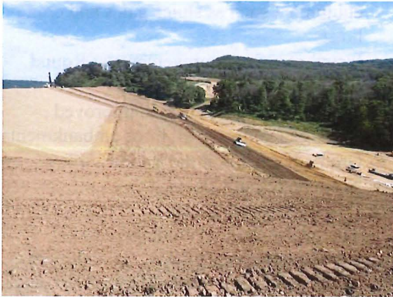
Topsoiling, seeding and erosion control mats being installed at the South Dam. Major earthwork was completed in August 2023.
