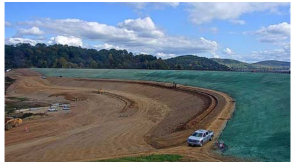
Major earthwork has been completed at the Round Valley Reservoir Dike Embankment. Restoration work including placement of topsoil and hydroseeding is being conducted.
