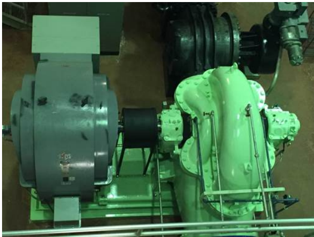
South Branch Pump Station 2000-HP pump, motor and baseplate after 2016 rehabilitation
