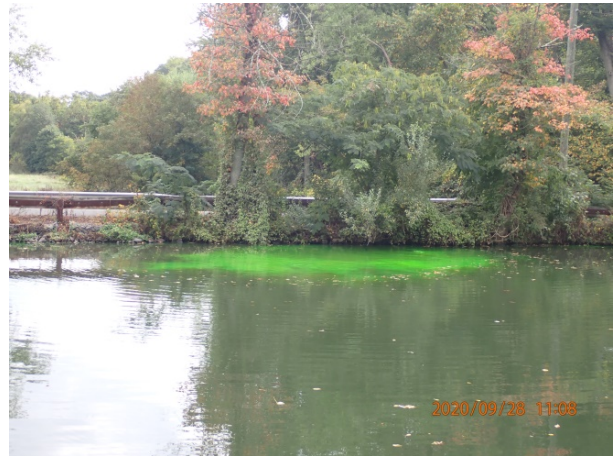
Dye testing for leaks being performed in canal above the Six Mile Run Culvert.
