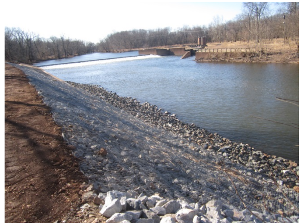
Stabilized embankment between Raritan River (Right in photo) and D&R Canal with gabions and rip-rap downstream of the Island Farm Weir (weir in background)
