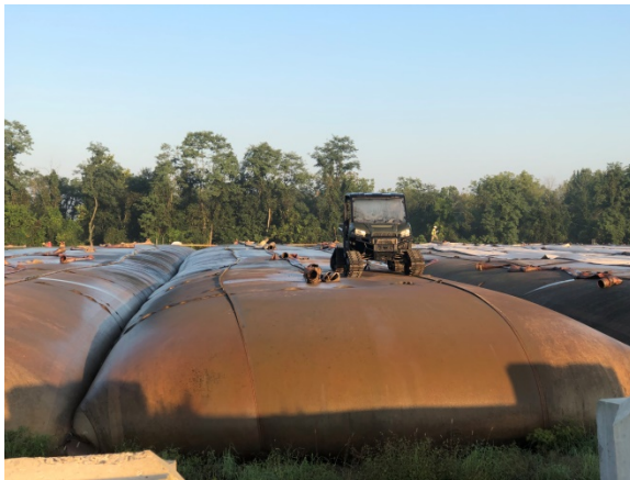
Geobags in drying (staging) area during dredging operations. Silt-laden water is directed to the geobags that filter the sediment. Clean water is discharged back to the Canal.
