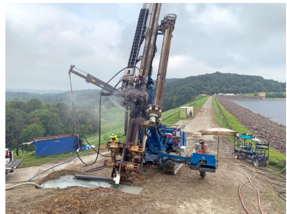
Drilling work occurs on the left abutment of the South Dam during the Round Valley Reservoir North and South Dam Abutment Grouting Project.
