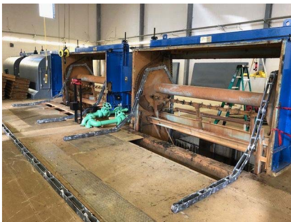
Disassembled traveling water screens
