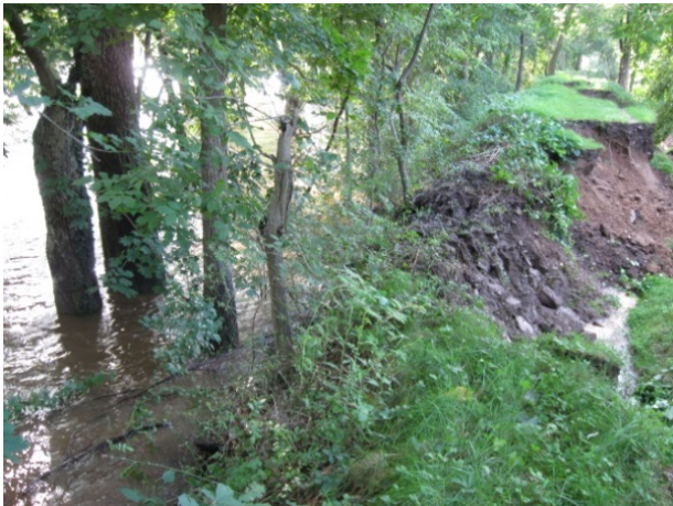
D&R Canal embankment in Stockton Borough in 2011.
