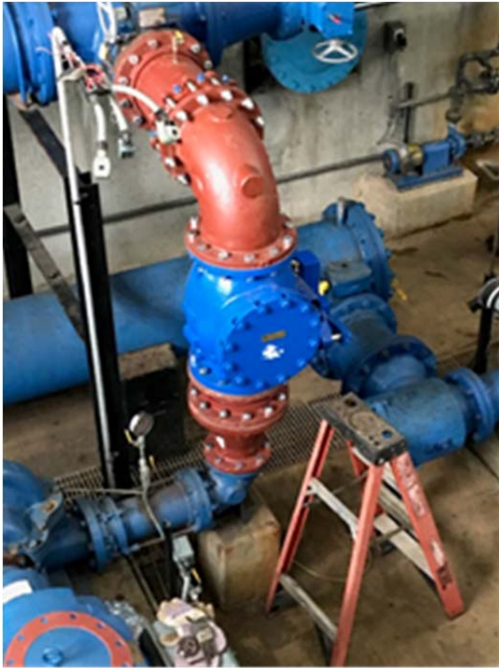
Example of one of the piping and valve replacements at the MWTP. Photo taken before painting.
