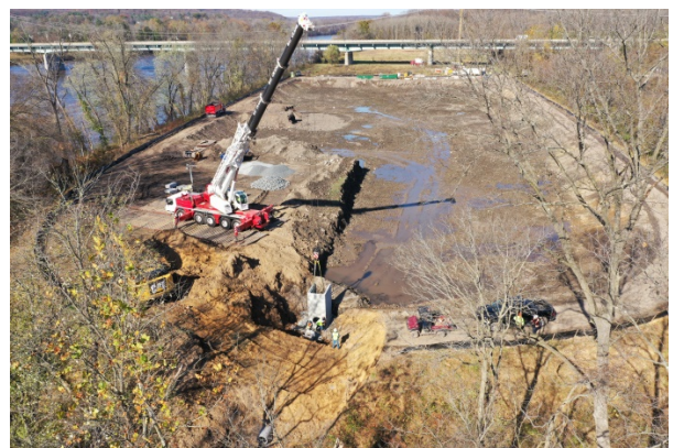
Overhead view of Route 202 Stockpile area in Delaware Township New Jersey during trucking operation. Crane on site to place new dewatering structure.
