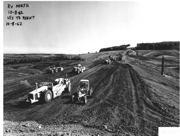
Round Valley North Dam under construction, October 1962. What is now the reservoir would be to right in photo.
