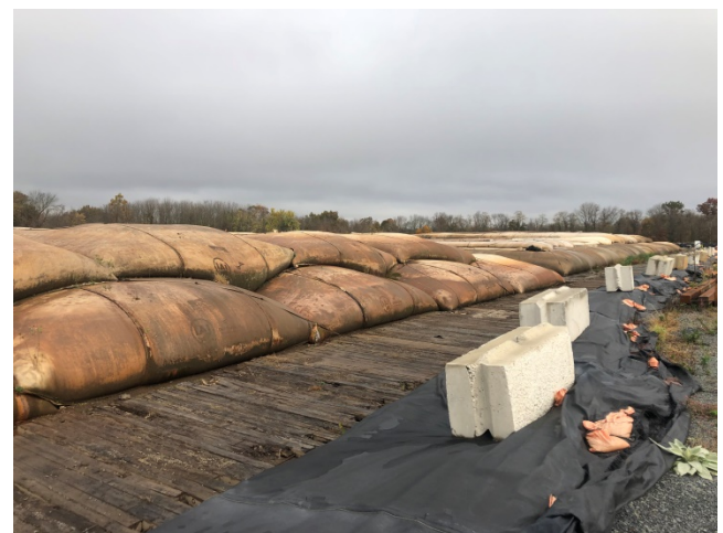
Geobags in drying (staging) area during dredging operations. Silt-laden water is directed to the geobags that filter the sediment. Clean water is discharged back to the Canal.
