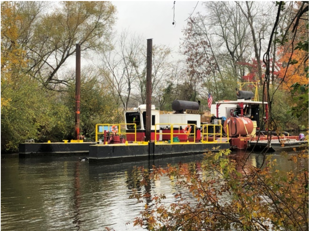
“Fox River” Dredge, one of two dredges working in 2019. Note the boom extending into water in front of dredge in photo. Note three vertical square “spuds” keep equipment in place while dredging. Square plates at base of “spuds” prevent damage to clay liner at bottom of Canal. On-board computer and GPS maintain location and depth of boom and cutter head to prevent damage to the clay liner.
