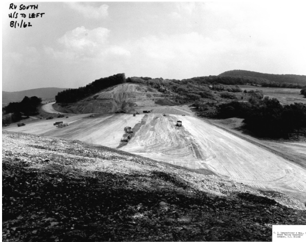
Round Valley South Dam under construction, August, 1962. What is now the reservoir would be to the left in photo.
