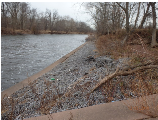
Note erosion of embankment between Raritan River (left in photo) and D&R Canal just downstream of Island Farm Weir.
