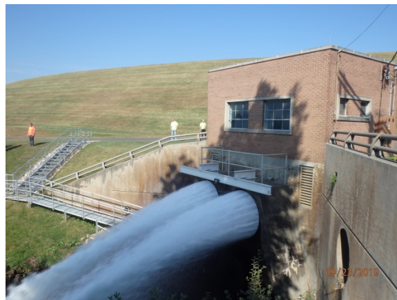
Spruce Run Vault. Howell Bunger Valves in Operation.
