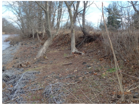
Note erosion of embankment between Raritan River (left in photo) and D&R Canal just downstream of Island Farm Weir.
