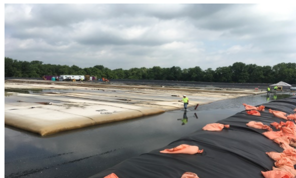
Geobags in constructed drying (staging) area during dredging operations. Silt-laden water is directed to the geobags that act like a filter. Clean (elutriate) water is discharged back to the Canal.
