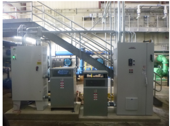
Variable speed controls for Motors at the MWTP
