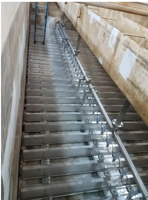
Underdrain at filter support laterals at the MWTP
