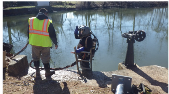
10-Mile Waste Gate was replaced “in the wet.” After flow through the gate was temporarily stopped on the river side of the structure, the gate was replaced without dewatering. In this photo, a diver enters the water to perform work on the replacement gates.
