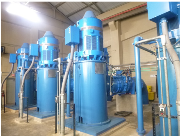
Variable speed motors on reservoir fill pumps
