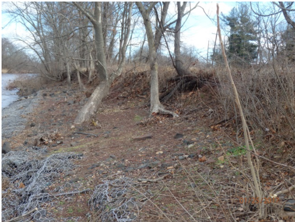
Note erosion of embankment between Raritan River (right in photo) and D&R Canal just downstream of Island Farm Weir.
