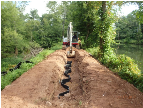
Steel sheets cut down to size will eventually be backfilled below grade. Canal to right in photo. Millstone River to the left.
