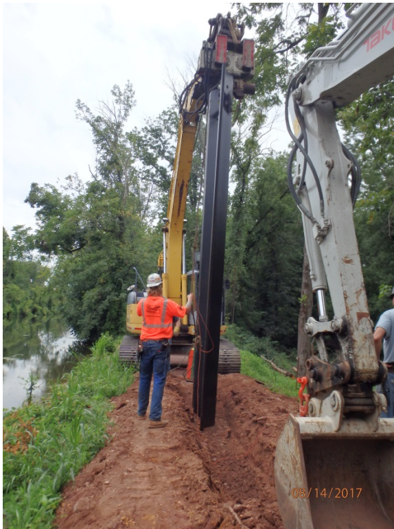
Contractor driving steel sheets down centerline of towpath. Canal to left in photo. Millstone River to the right.
