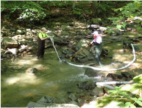
Sand Wand™ sediment removal system in use at the Spruce Run Inlet.
